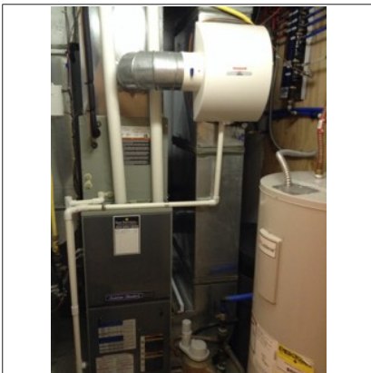
Utility room, main water shut off next to water heater
